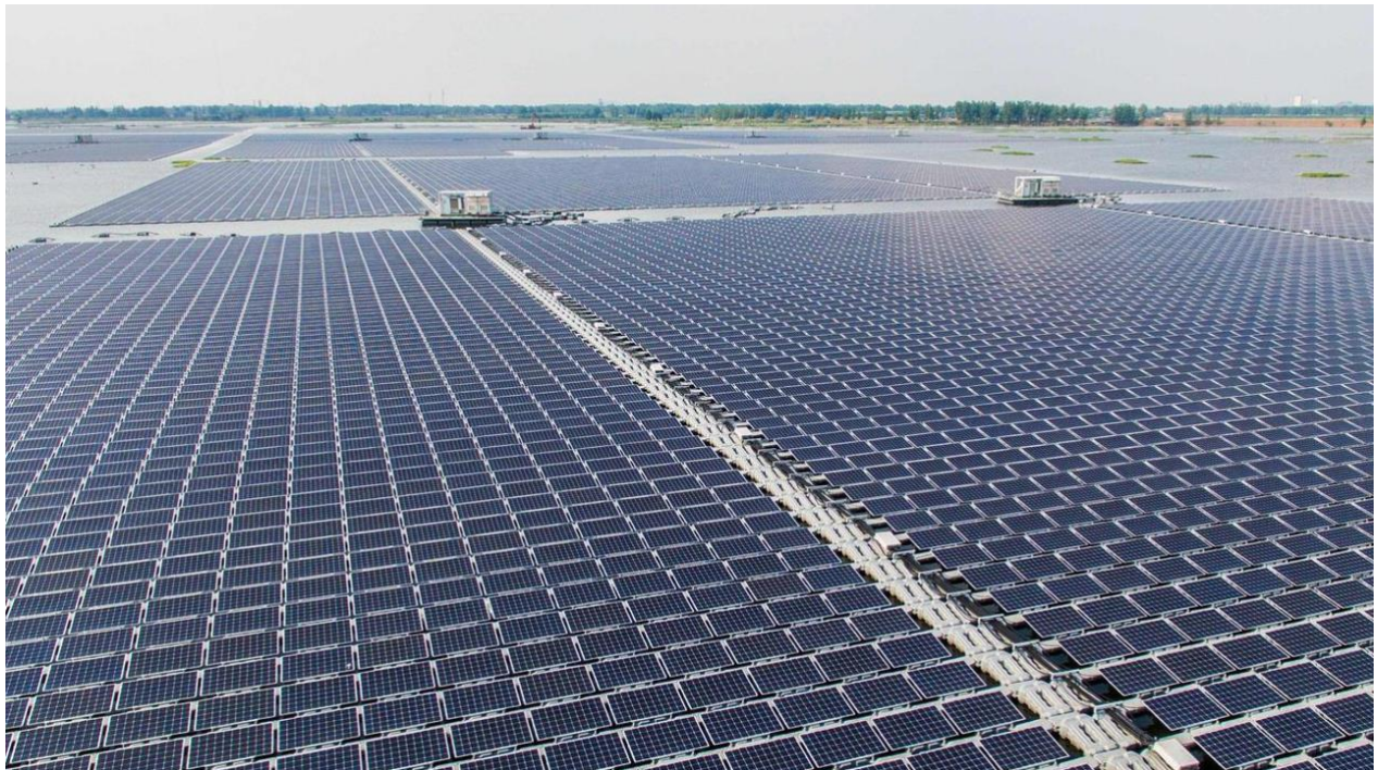
This solar farm in China's central Anhui province was the world's largest floating solar power plant in 2017. It has since been overtaken by multiple projects in China.
